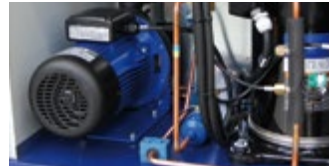
Pump P3 (3 barg) / P5 pump (5 barg, optional).
